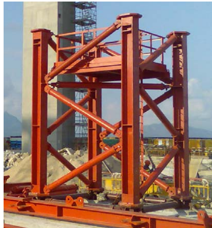
Base mounted on concrete foundation.
